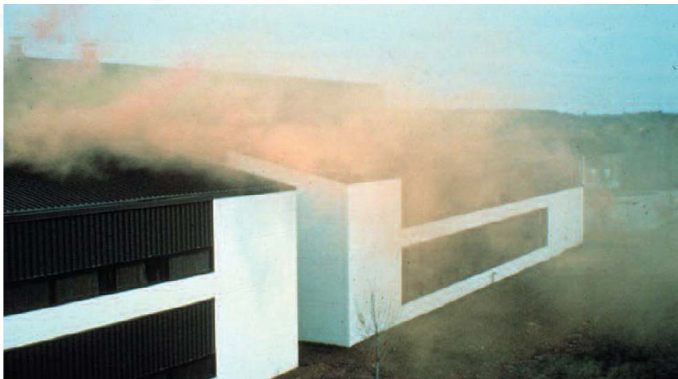
Often, exhaust streams are re-entrained at outside air intakes without anyone knowing. In this photo, colored dye shows just that.
