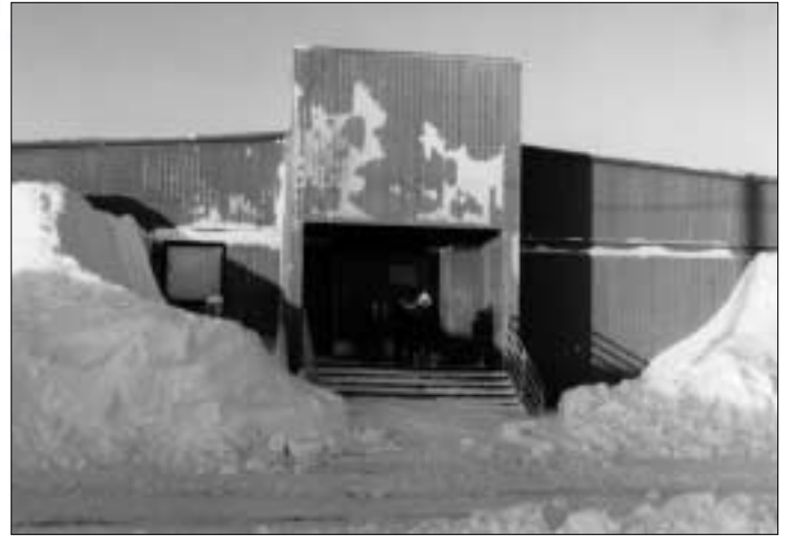
Snow drifts form on either side of the entrance because of the wind deflector over the doors.
